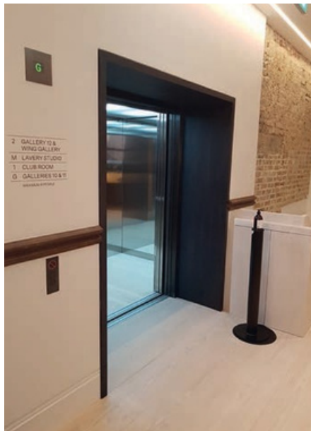
Passenger and goods lift for transportation of people and items to all floors
