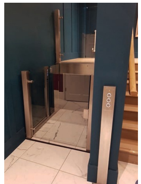
A stylish, modern scissor lift installed in the hotel reception for visitors with impaired mobility
