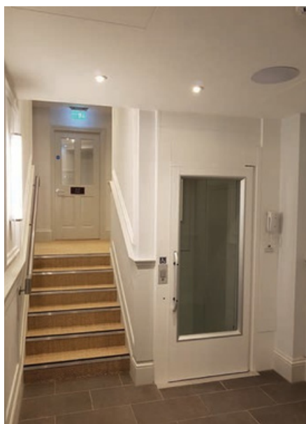
Platform lifts allow easy movement between small floor level differences within the hotel
