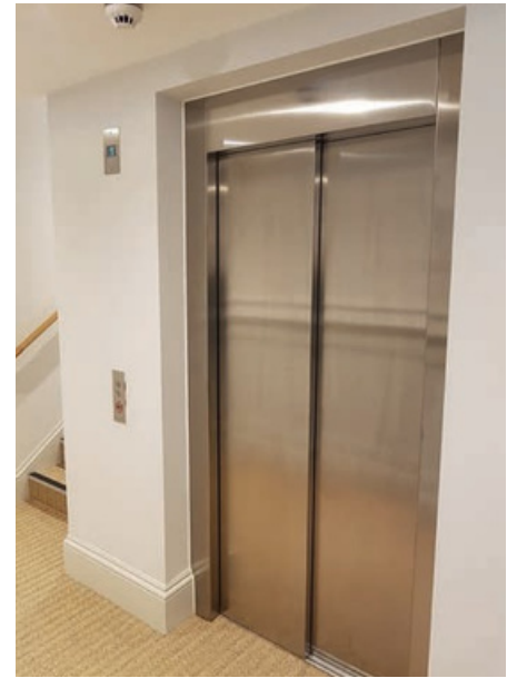
Passenger lift installed with a bright stainless steel finish for all fittings and landing doors
